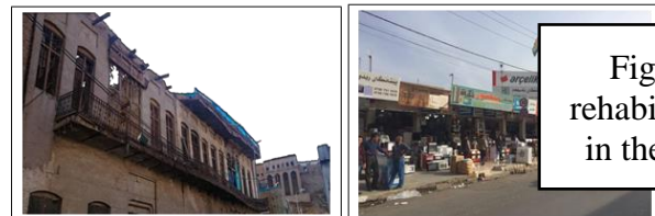
Figure (11) The lack of building controls for the organize the uses and visual pollution, in addition to distortion of building elevations
