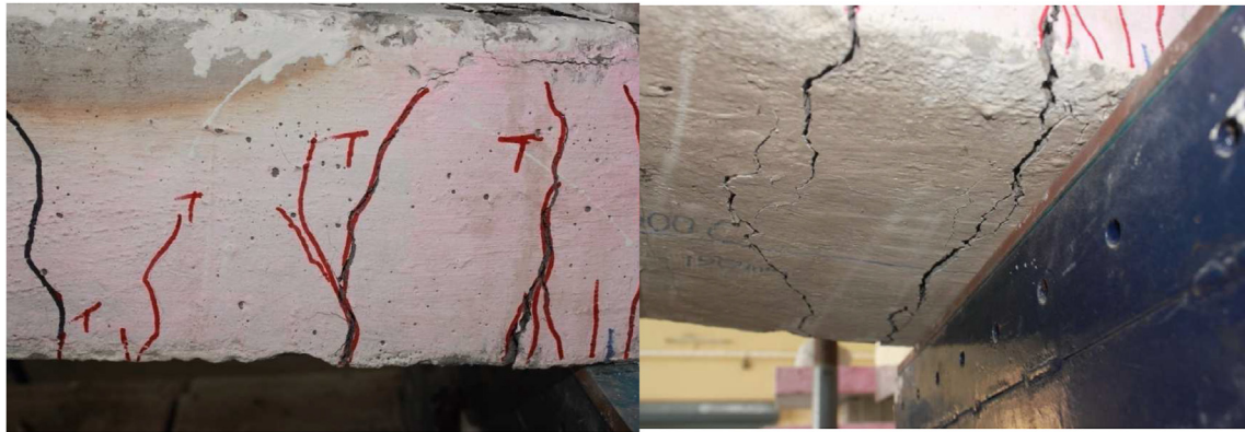
a) Cracking of Specimen in the tension zone under mechanical loading
