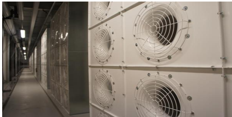
15 motors per server bank
