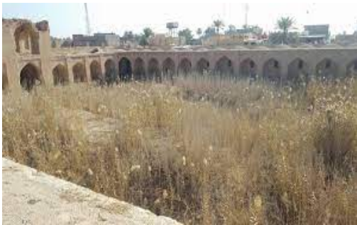
Neglect, some parts are destroyed and debris is accumulating Source: Google image 4
